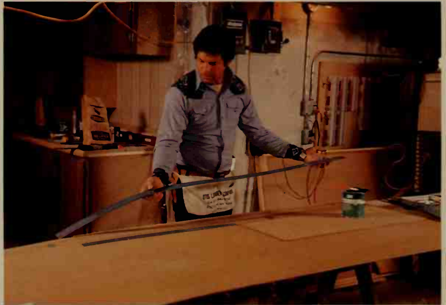
Cutting a strip of plastic laminate, the carpenter applies contact cement and attaches the strip to the counter edge.
