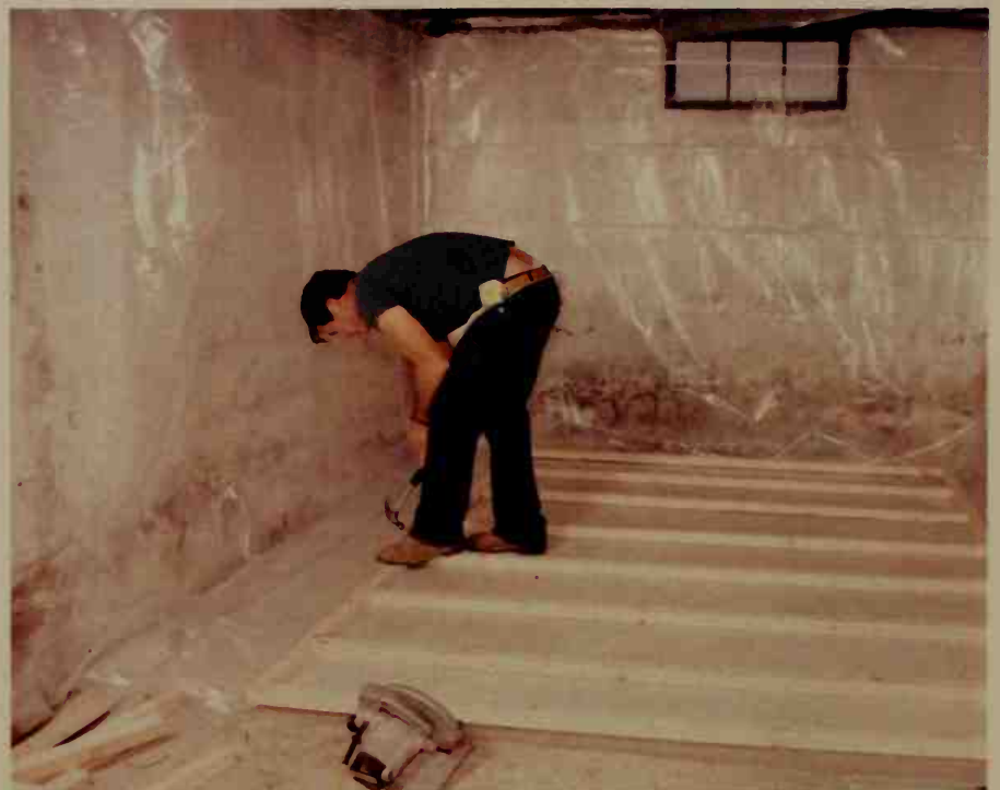
The easiest way to construct the wall furring is to assemble the 2 x 2s on the floor and then raise the whole wall unit into place.
