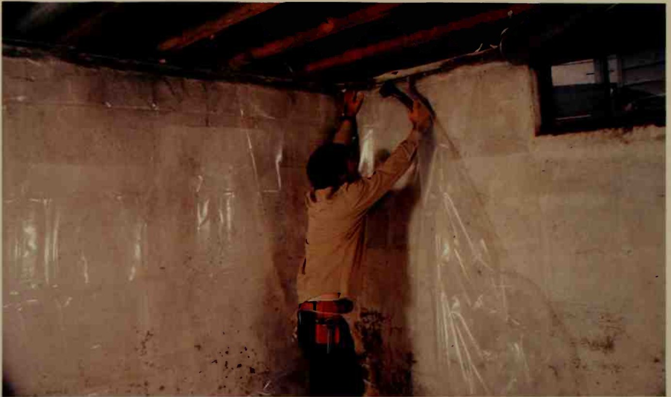
Since this is a basement room, we are providing a vapor barrier of plastic sheeting to minimize any moisture problem.
