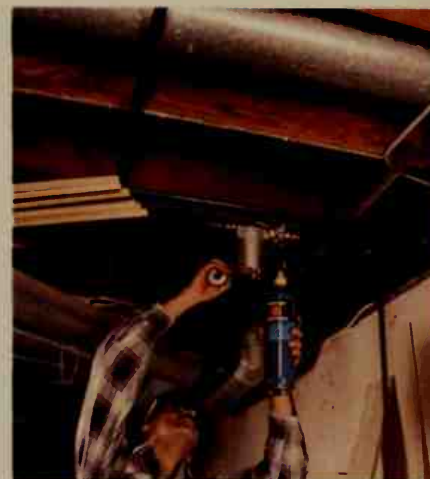
As we reconstruct the water lines, we are adding a filter to the supply line.
