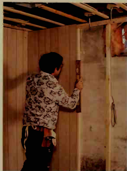
Only when all of the electrical and plumbing connections are complete, can we install the paneling.
