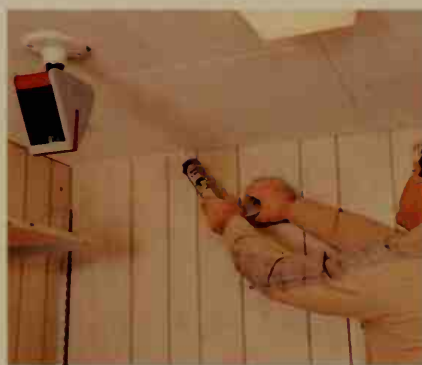
To make sure our darkroom does not allow stray leakage of light or air we caulk seams carefully.
