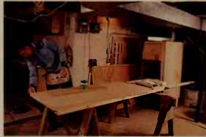
When he has prepared the counter top with double-thickness particle board at the edges, our carpenter prepares the edge surface with contact cement.
