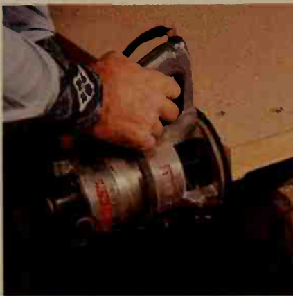
The carpenter uses a router with a special bit to trim and bevel the excess laminate (left deliberately so that slight misalignment is not critical).
